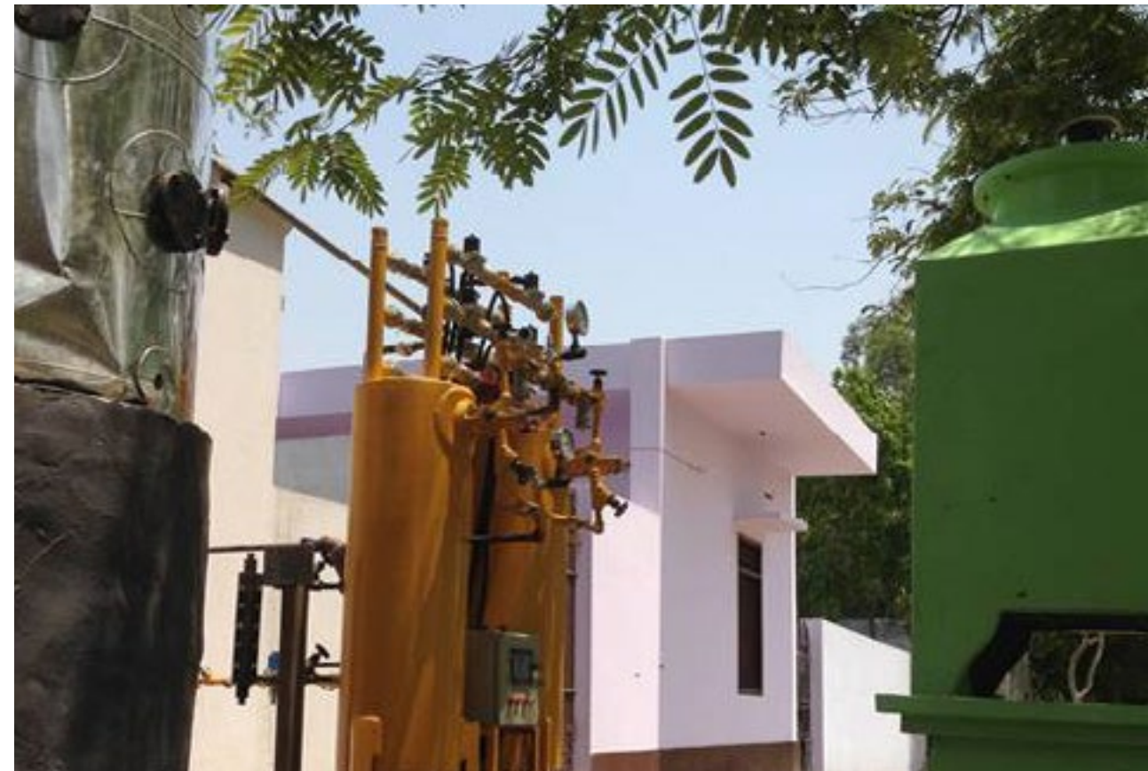
The GreenCHILL biogas-powered refrigeration system cools a 10 metric ton cold storage unit. Photo courtesy of GreenCHILL.
